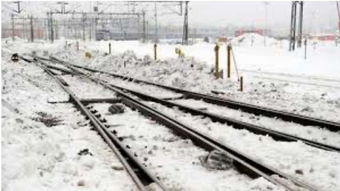
Figure 4. An electrically heated railway switch under winter conditions (SVT Nyheter 2019-02-09)
