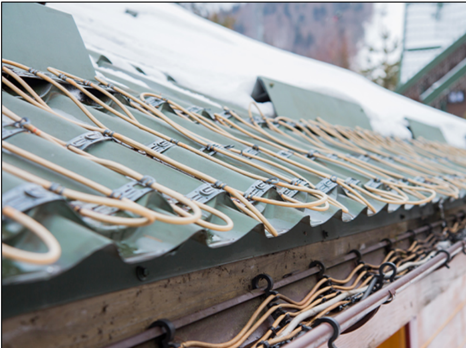
Figure 3. Electric cables are commonly used for snow and ice on roofs and roof dewatering systems (Photo: Värmekabel Stockholm AB 2023).
