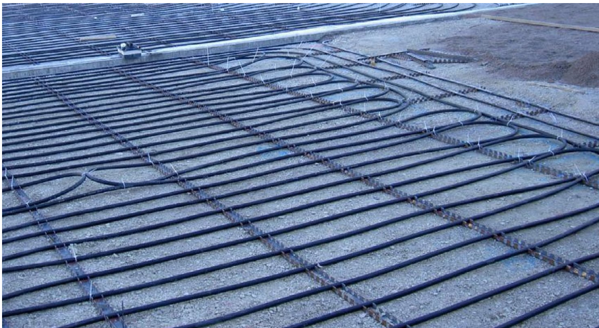
Figure 13: PE pipes placed directly on the ground and fixed by specially made guides (LK Systems)
