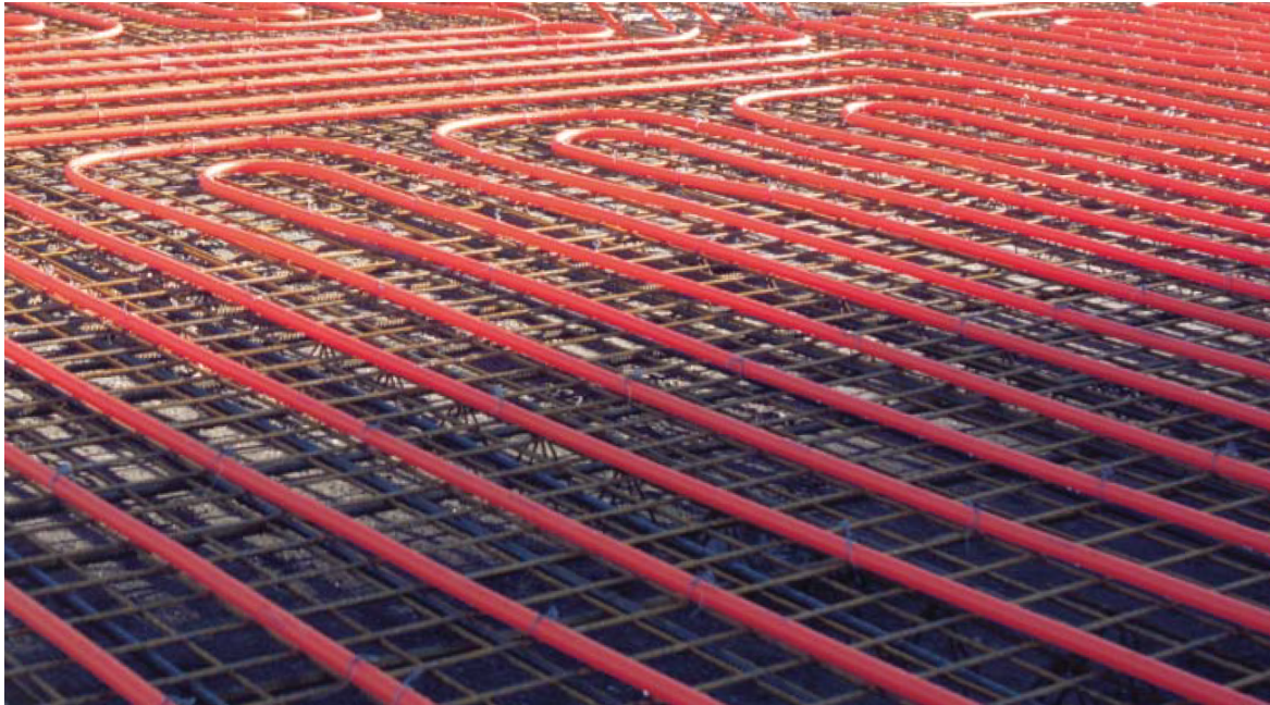
Figure 12: Part of a surface with PEX pipes fixed to a mesh of rebar and ready to be cast into concrete (Uponor)
